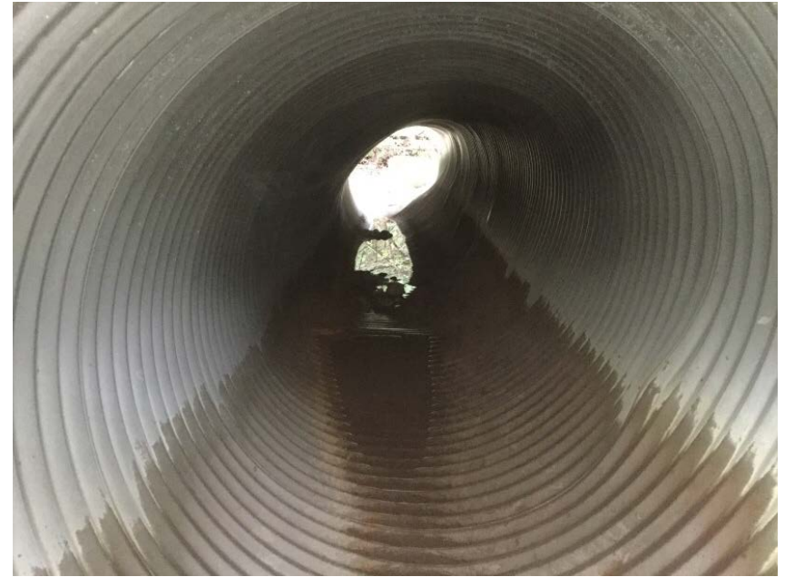
Damage to roof of right culvert
