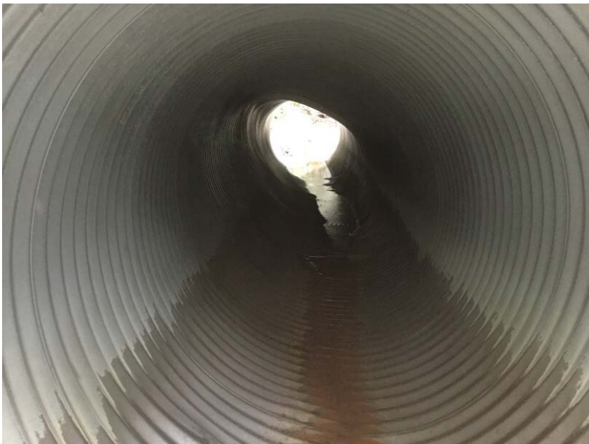
Damage to roof of left culvert
